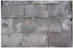
Example of: Slate Wall Shingles / Cladding (Photograph indicative) Roofing slate installed as rainscreen cladding on vertical external walls.
